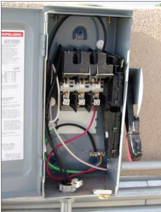
Photo 7. Line and load connections are important
