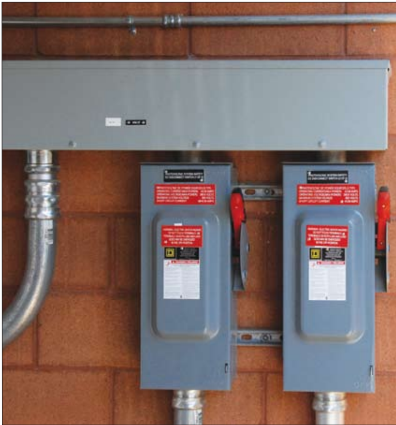
Photo 5. PV dc disconnecting means
