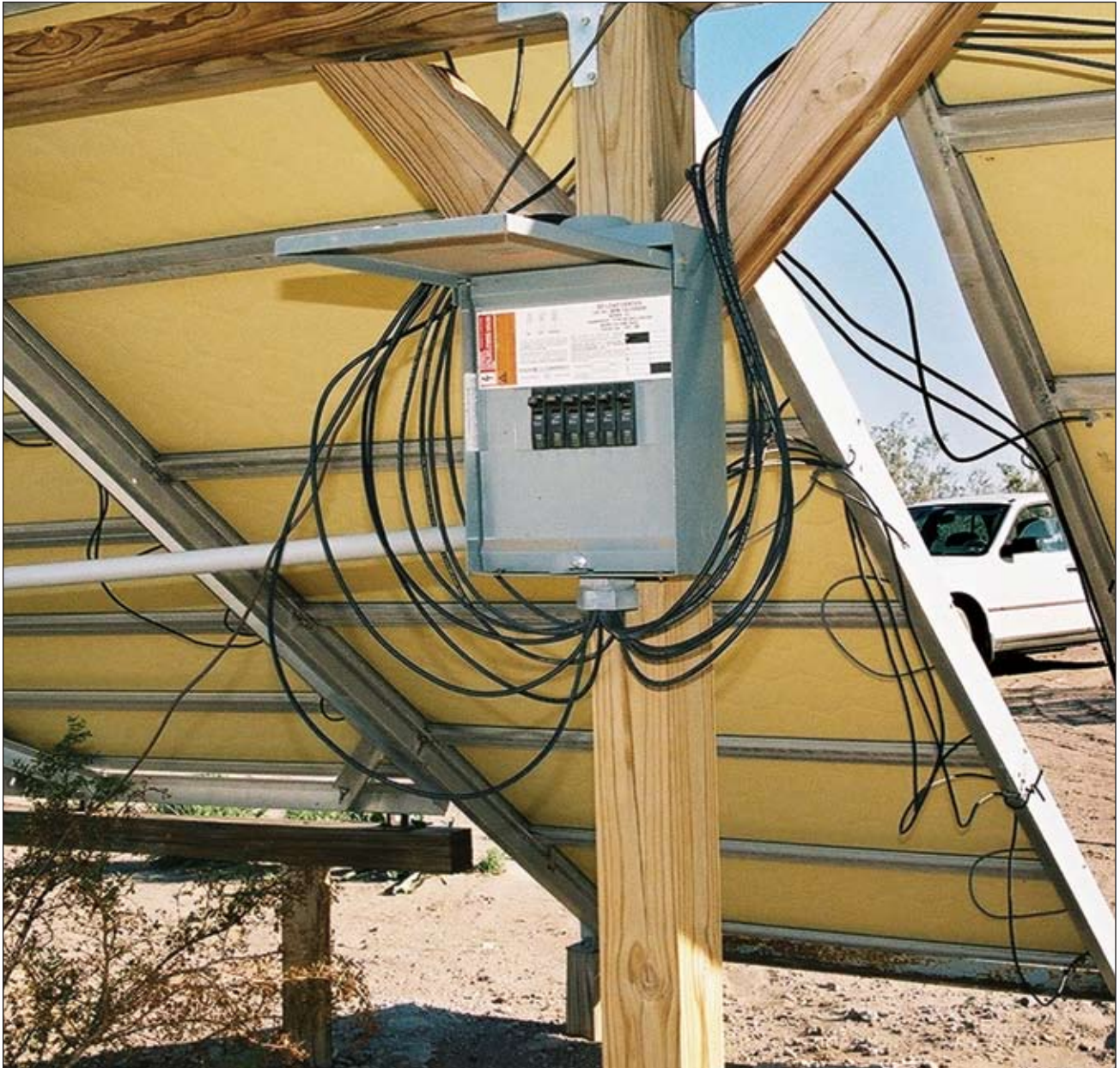
Photo 2. PV source-circuit combiner with circuit breakers—poor workmanship
