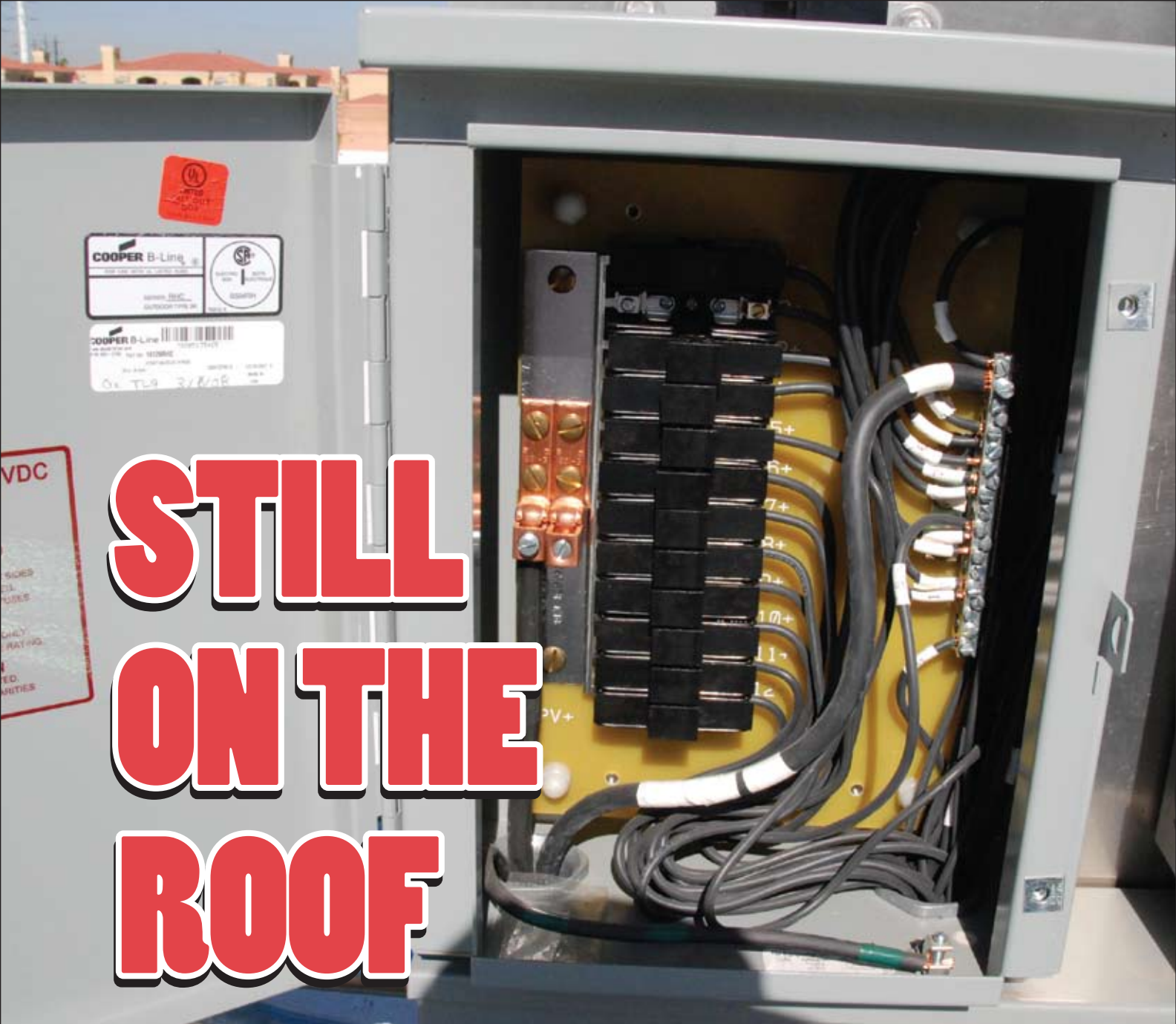
Photo 1. PV source-circuit combiner with fuses
